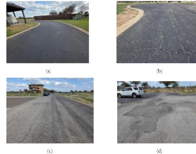
Figure 3. Common Distresses: (a) Longitudinal and Transverse (LT). (b) Block Cracking. (c) Weathering and Light Raveling. (d) Localized Patching.
